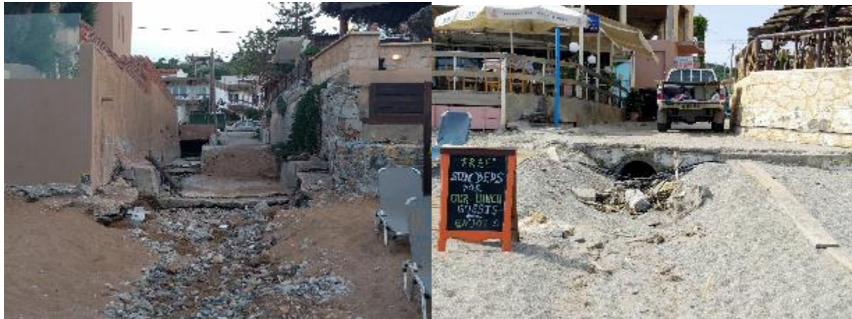
Figure 49. Observed beach conditions showing significant erosion and debris due to runoff from channels
