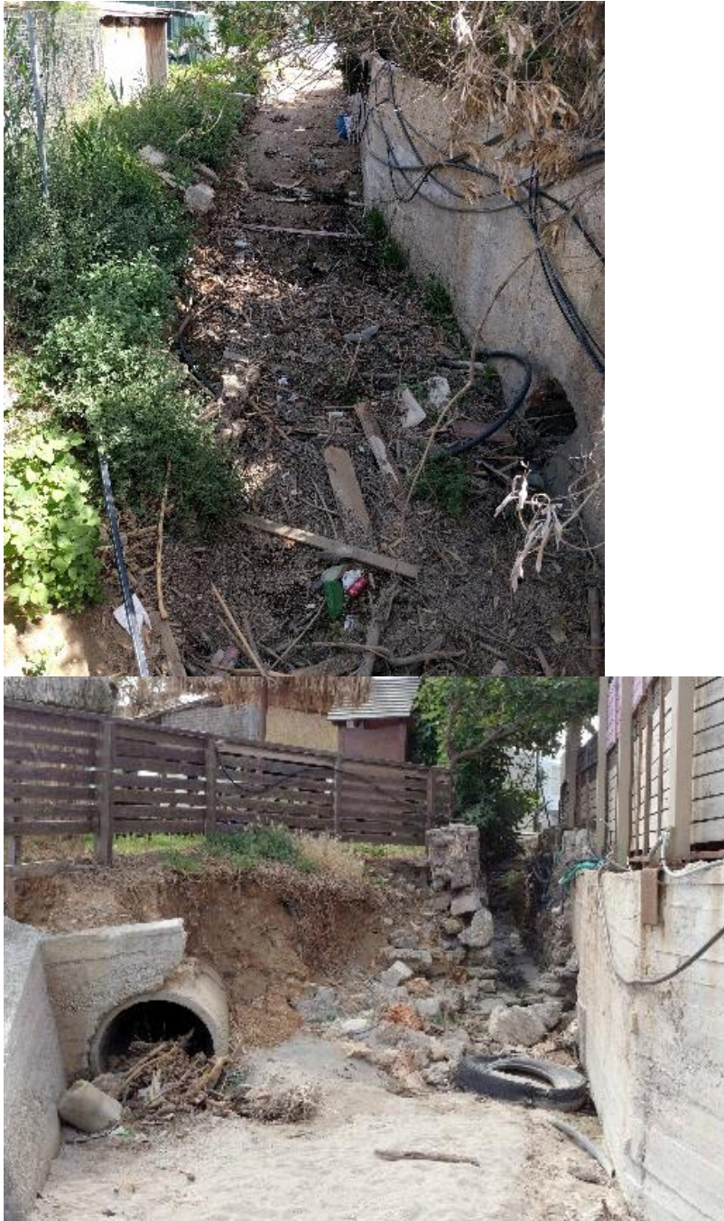
Figure 74. Many of the channels in the study area are full of trash and poorly maintained
