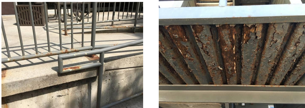
Figure 25. Metal elements in need of repair
